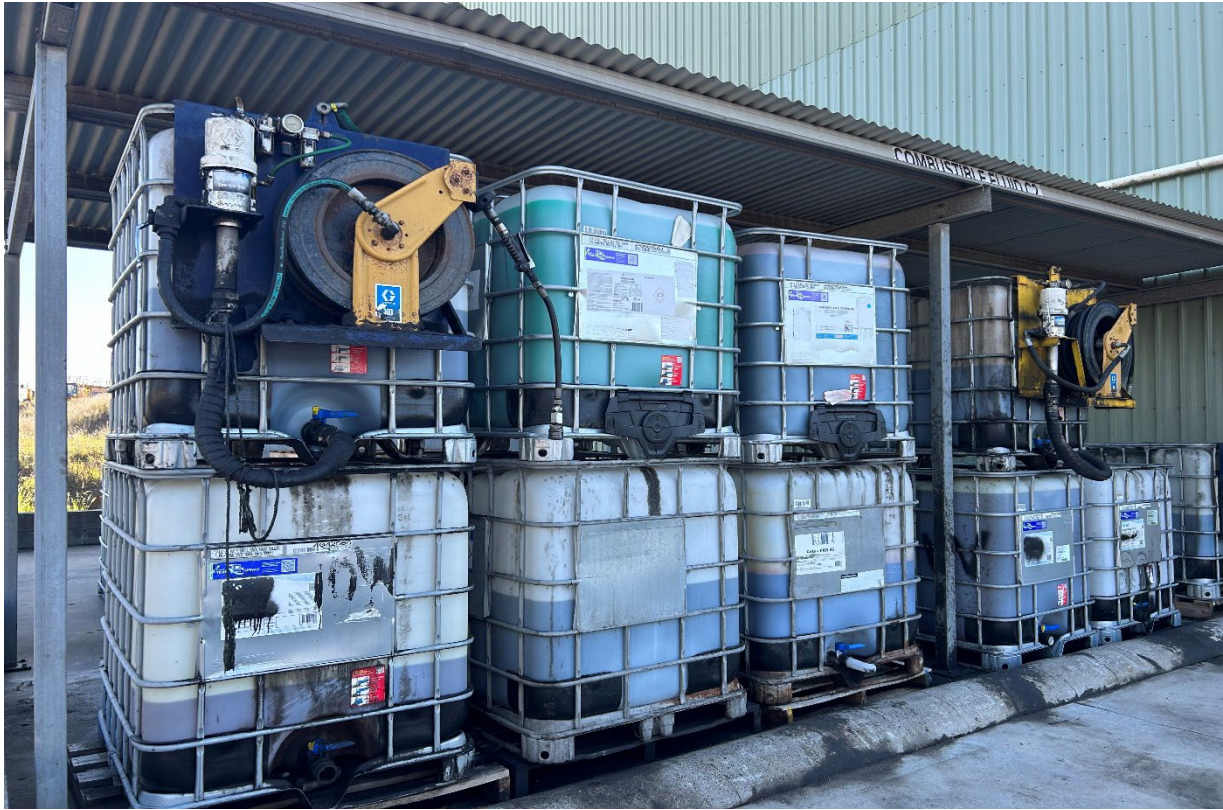
Plate 13 – Bunded chemical storage area
