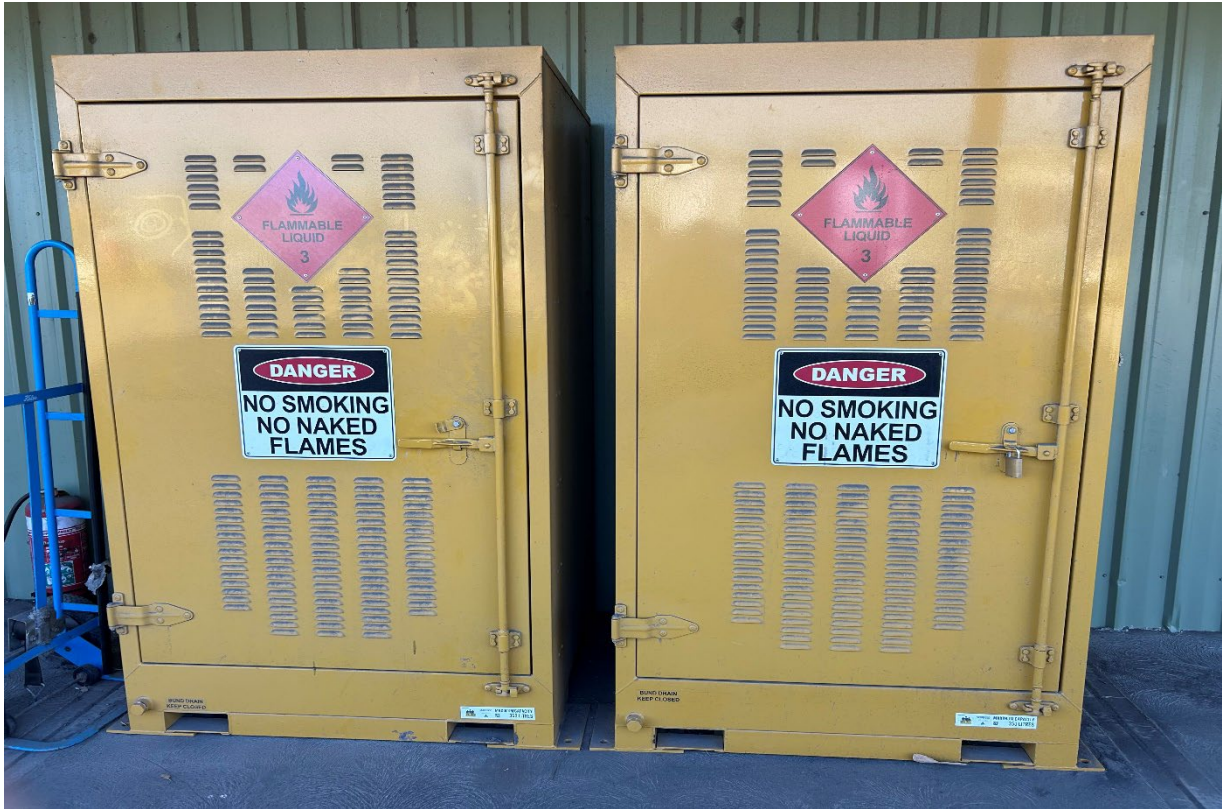
Plate 11 – Flammable liquid storage
