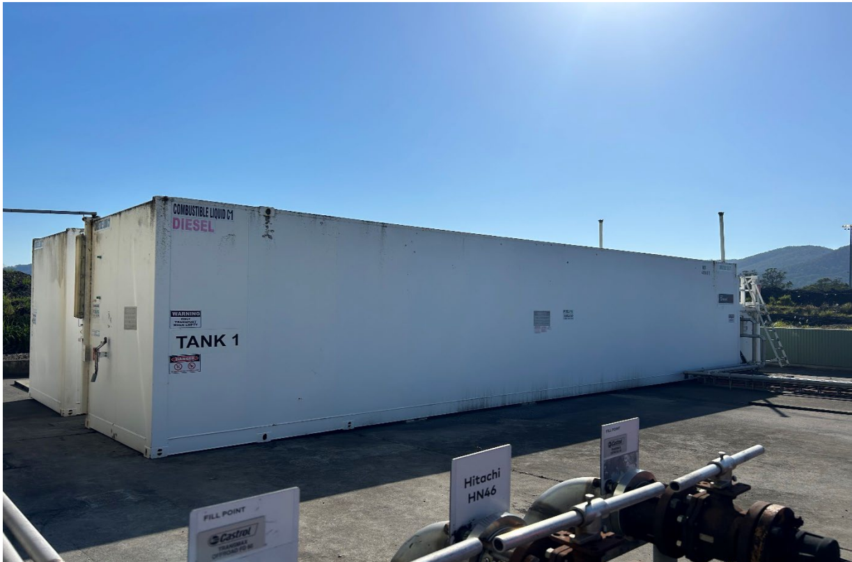
Plate 14 – Bunded diesel tank storage area
